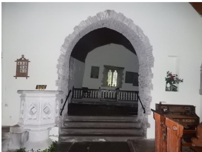
Photo 3271: chancel of Cwmyoy Church, showing the distortion
